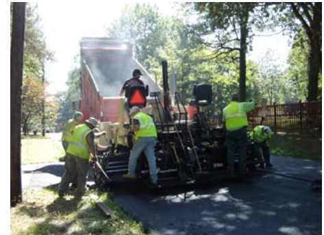
Woodbridge Township Public Works "road paving crew" complete paving Avalon Drive and the Harrow Street Drive entrance to Colonia High School. The paving program is part of a shared services initiative announced by Woodbridge Mayor John E. McCormac and Superintendent of Schools Vincent Smith.
